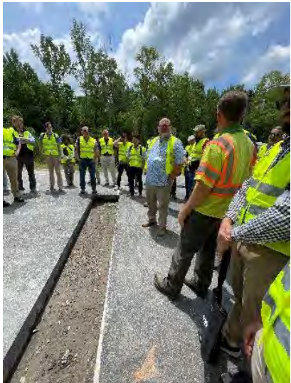
Figure 1 NCAT Cold Central Plant Recycled Mix Test Section sponsored by VDOT. No cracking after 30 million ESALS.
